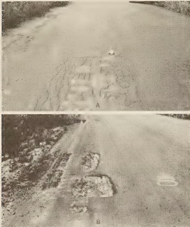
FIGURE 10.—PLACES WHERE SURFACE FAILURE OCCURRED. A, THE RECTANGULAR PORTION IN THE CENTER WAS REMIXED AND TAMPED BY HAND; SHINY AREAS ARE POOLS OF BITUMEN. B, BREAK-UP CAUSED BY UNTREATED SAND LYING BETWEEN UPPER AND LOWER PORTIONS OF THE MAT.
